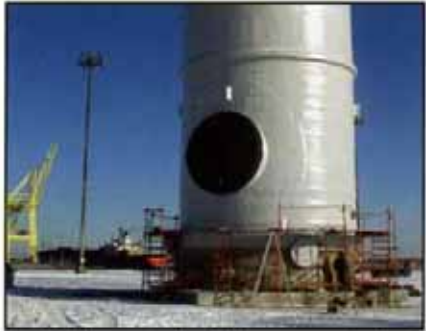
Steel blinds were made to allow pressure testing of the scrubbers at the port.
