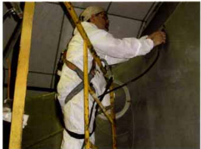
Plastic-welding to ASTM C-1147 specifications with a PVDF cap strip gives seams more tensile strength than the lining.
