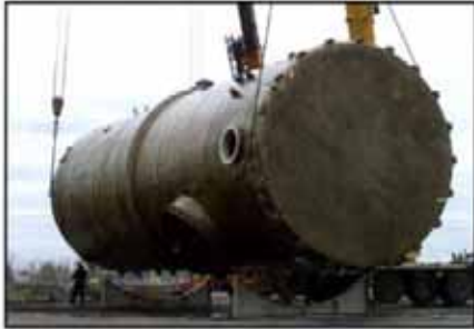
After assembly at the port, the scrubber is moved for pressure testing.
